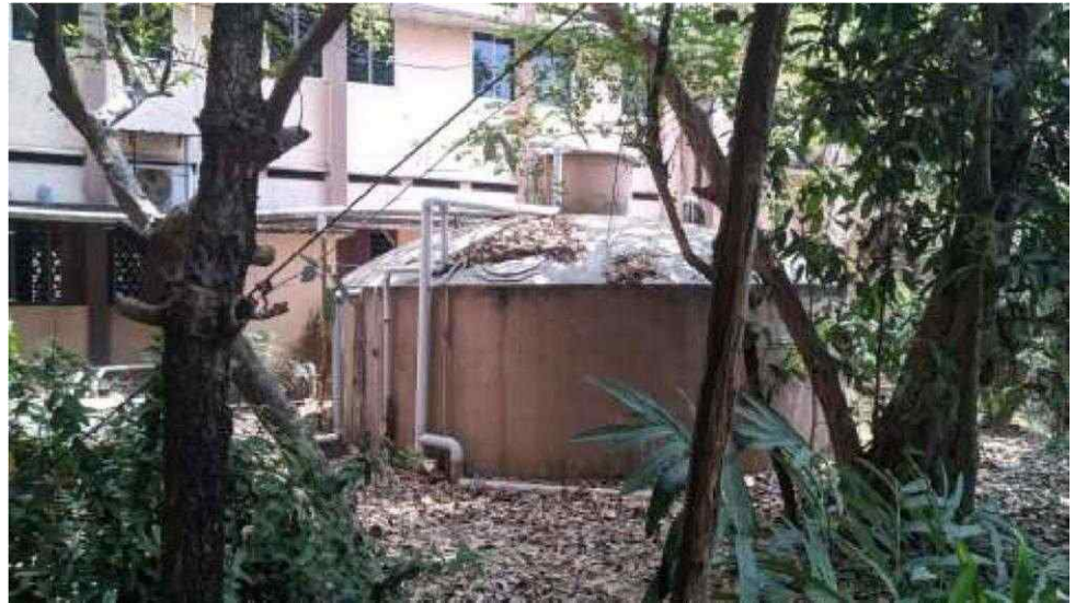
Fig. 4.5 Rainwater harvesting tank
