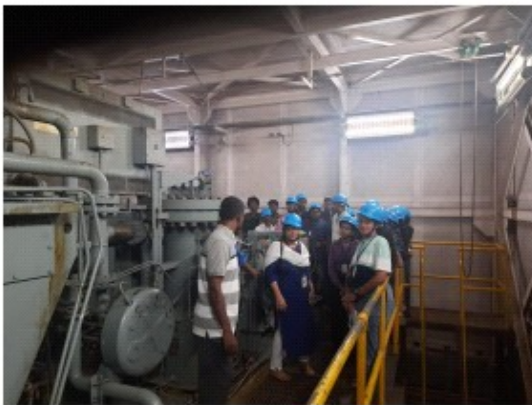
Photo 2: Inside of Thermal Power Plant
